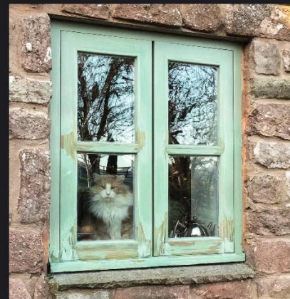
Old, flaking timber windows in need of updating and replacing
